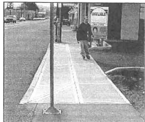
Driveway crossings with excessive cross slope
