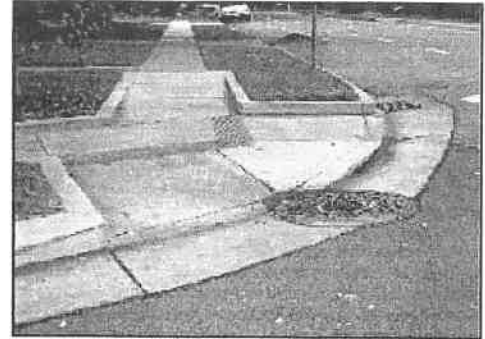
This curb ramp retrofit combines a parallel and a perpendicular ramp to stay within running slope limits. Curbed edges provide useful non-visual wayfinding cues. California State provisions (this is in Sacramento) require the corduroy markings at the intermediate landing, but research shows that the truncated domes required at the toe of the ramp (ADAAG 4.7) would provide a significantly more detectable indicator of the upcoming street crossing.
