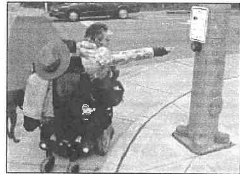
This new parallel curb ramp on a large-radius suburban corner curves down to the street and is otherwise usable, but the pedbutton isn't. Installed on a signal pole, it is out of horizontal reach range for this pedestrian. A better installation can be seen across the street, where a stub pole has been installed in a more usable location.
