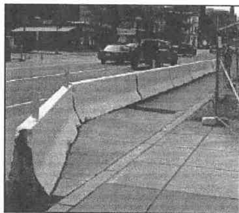
This urban arterial passes through a neighborhood that is undergoing rapid revitalization, with many projects under construction temporarily occupying existing sidewalk space. In this example, the contractor has provided a temporary pedestrian route in the curb lane of the roadway, separating it with Jersey barriers and installing a temporary concrete ramp to the street level walkway. Still needed: detectable warnings at the cross street.
